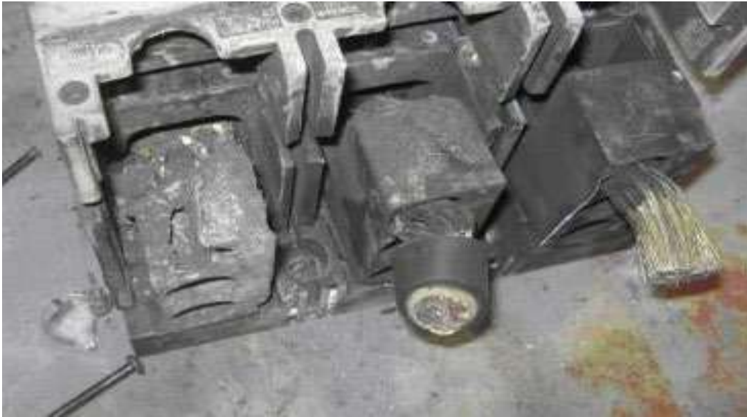
Damage to circuit breaker feeding a capacitor bank. A thermal examination would have detected abnormal heating
